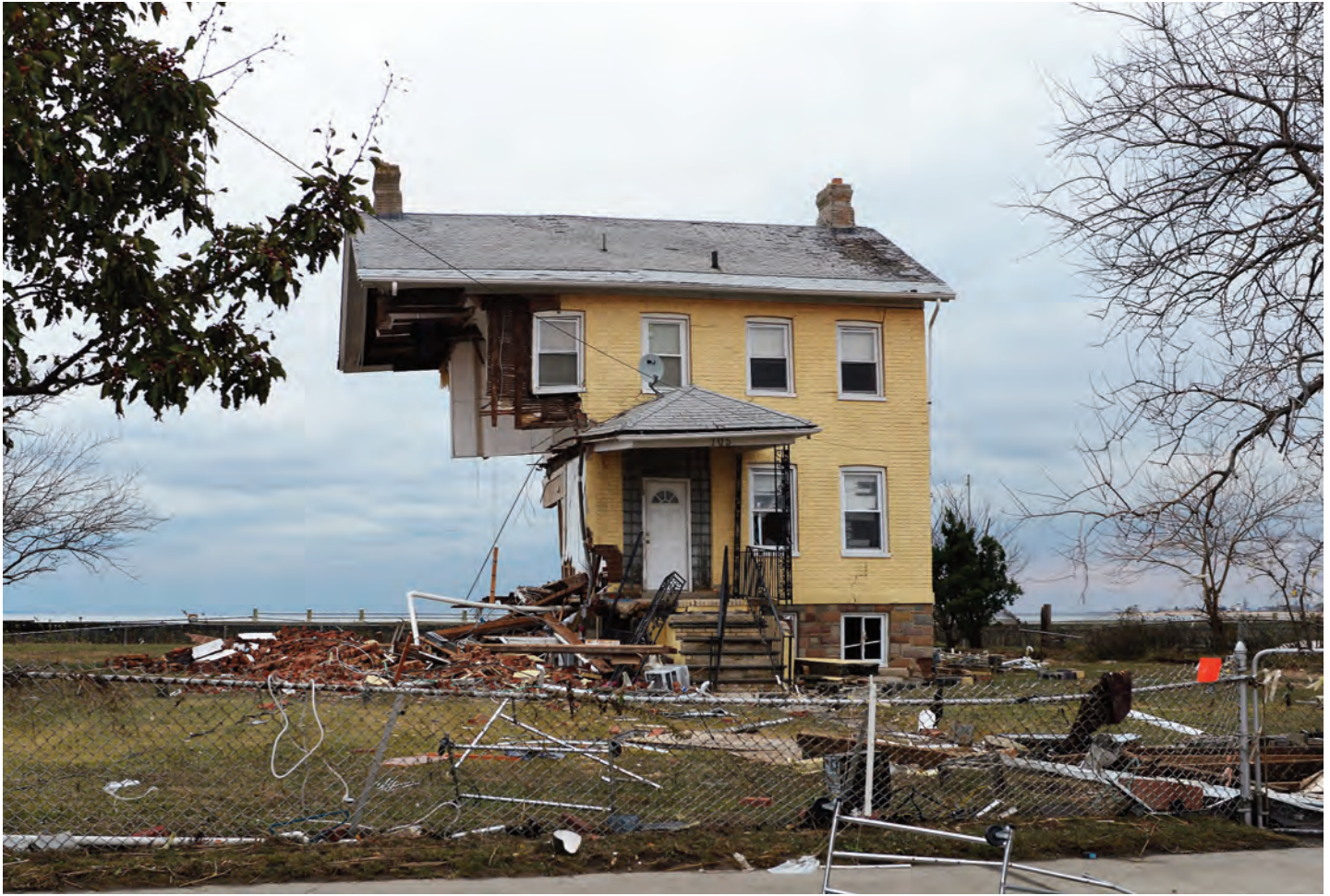
Hurricane Sandy was powerful enough to sweep away half of this brick house in Union Beach on northern New Jersey's Raritan Bay, including its masonry foundation, but curiously left undisturbed a satellite dish affixed to the roof of the building's porch. Photo: © Peter Massas via Flickr
