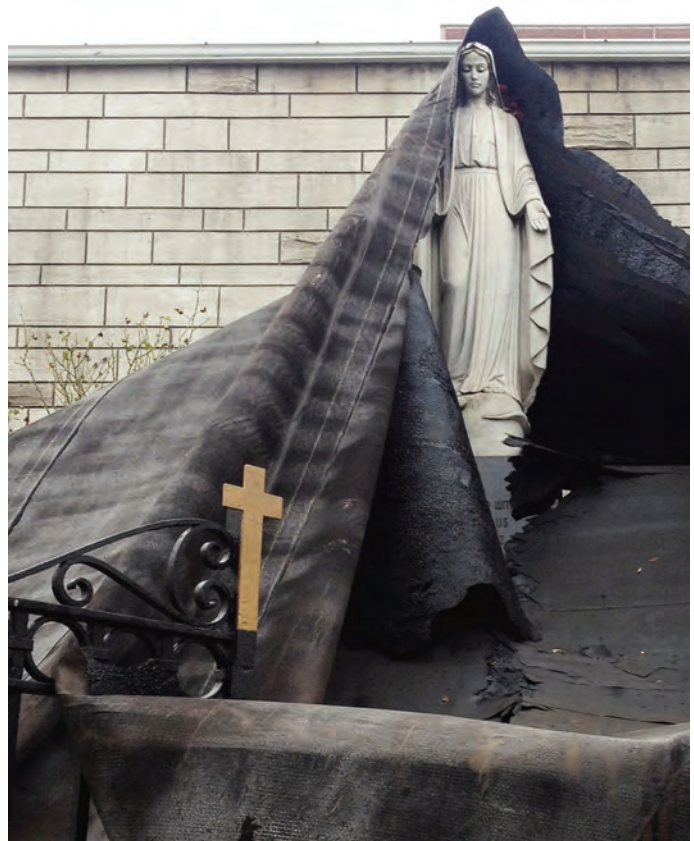
Roofing blown off a Jersey City, N.J., building wrapped around a nearby statue of the Madonna. Photo: © Sharla Sava via Flickr
