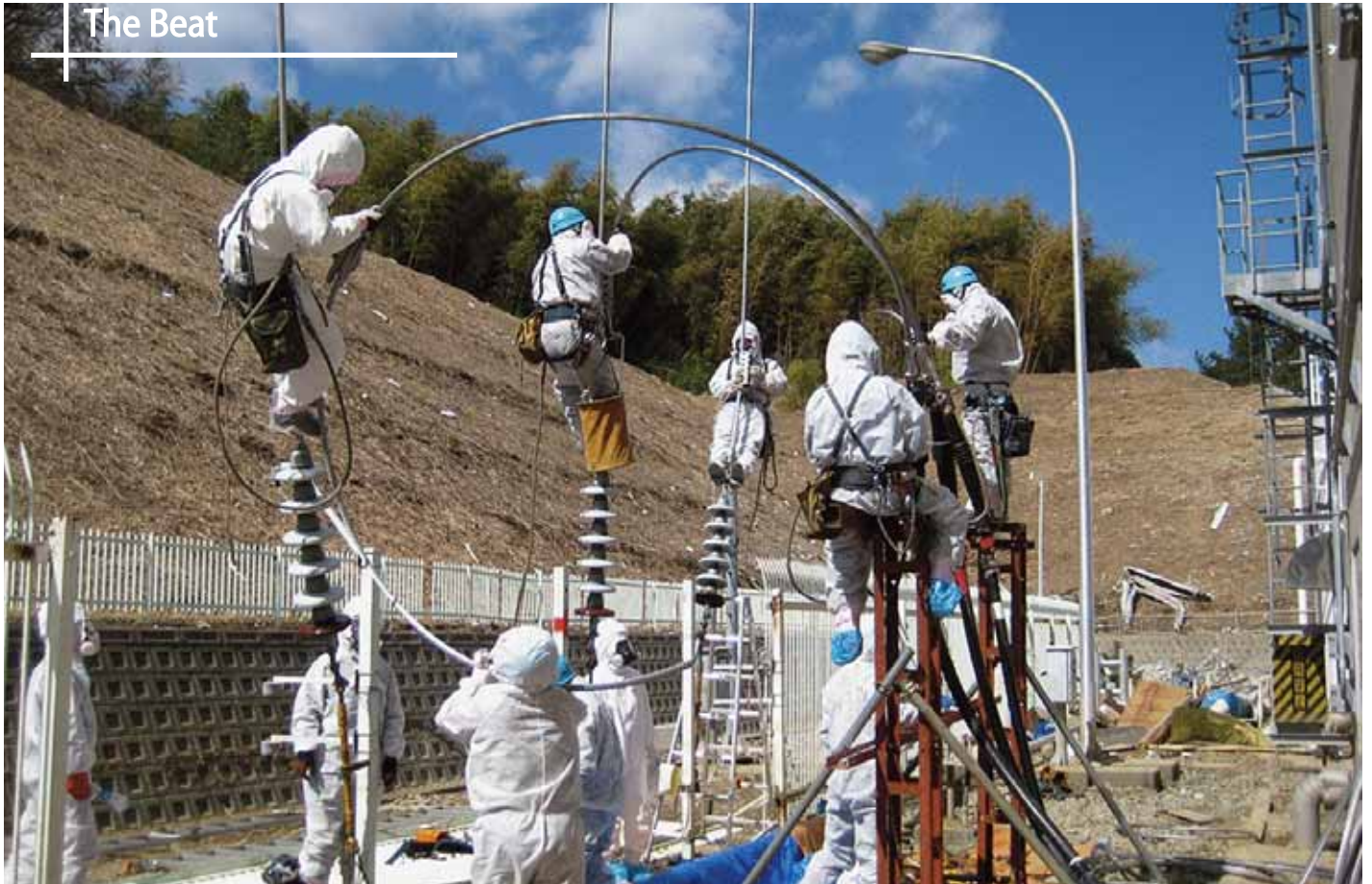
Workers connect transmission lines to restore electric power to the tsunami-crippled Fukushima nuclear power plant in Japan.
