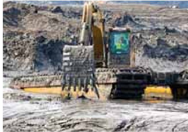
Amphibious trackhoes were used for clean-up operations in areas of the spill that were still too liquid to support large vehicles. Photo courtesy TVA.
