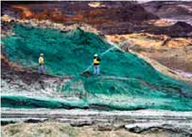
Clean-up workers spraying chemicals on the spilled ash to control dust. Photo courtesy TVA.
