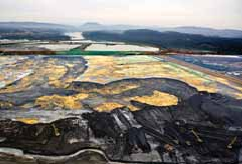
Aerial view of the cleanup of the remaining ash at the TVA Kingston Fossil Plant in Tennessee. Photo courtesy TVA.
